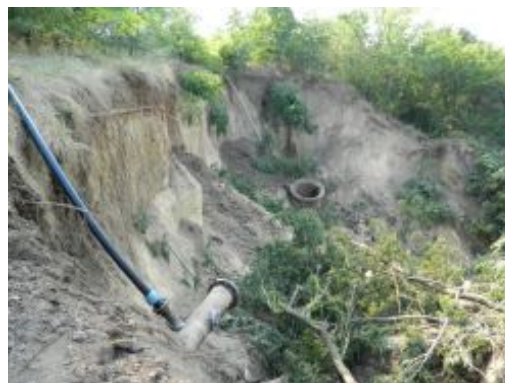
Fig. 2. Accident trunk sewer
