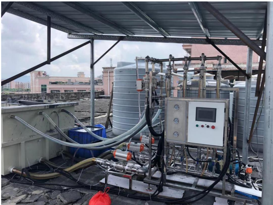
Figure 5.2 - Cutting fluid wastewater treatment
