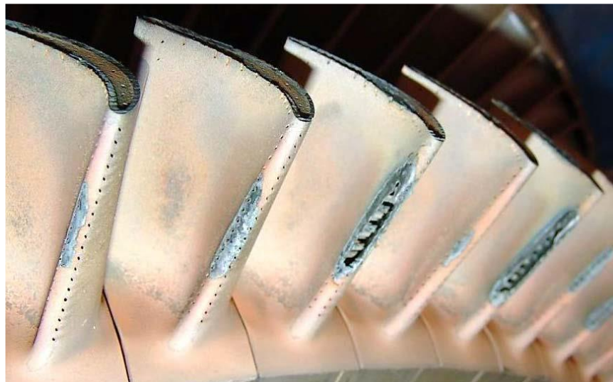
Рис. 3.7 Cases of burnout of gas-turbine engine blades, initiated by corrosion damage of the rotor blades of the first stage of the HPE
