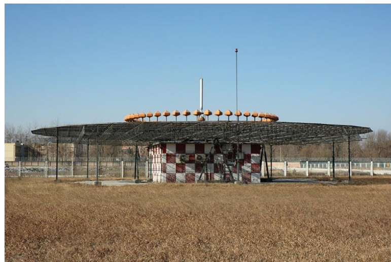
Fig. 3.2 – Ground station DVOR (Doppler VOR), combined with a DME transmitter
